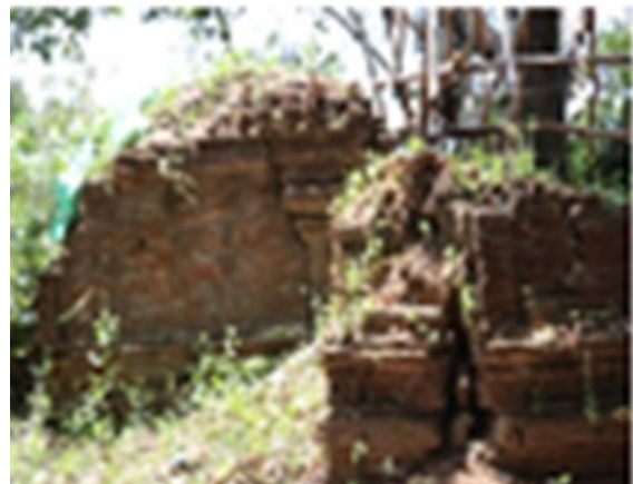
Figure 2: Damaged condition of Antharalam
